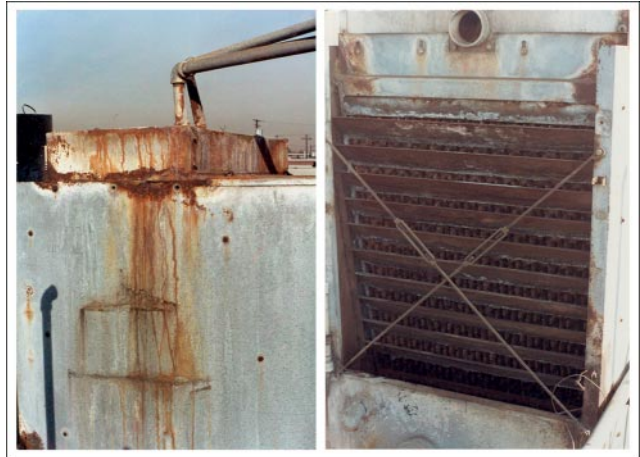
Metal-clad cooling towers are literally being eaten alive by harsh environments. They are attacked internally by process chemicals and externally by environmental elements.
